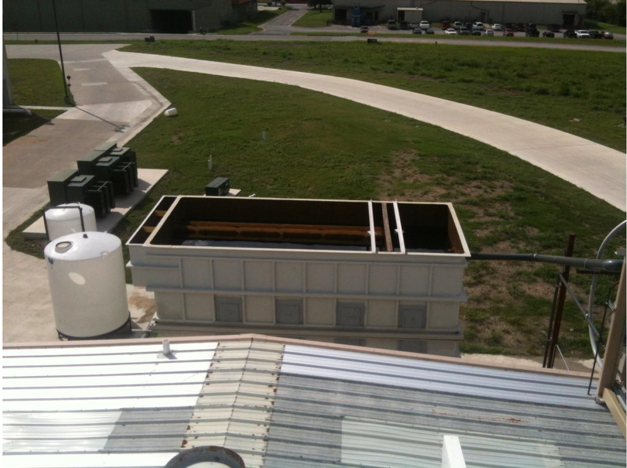
Figure 10. High performance clarifier installed after extended aeration tanks
