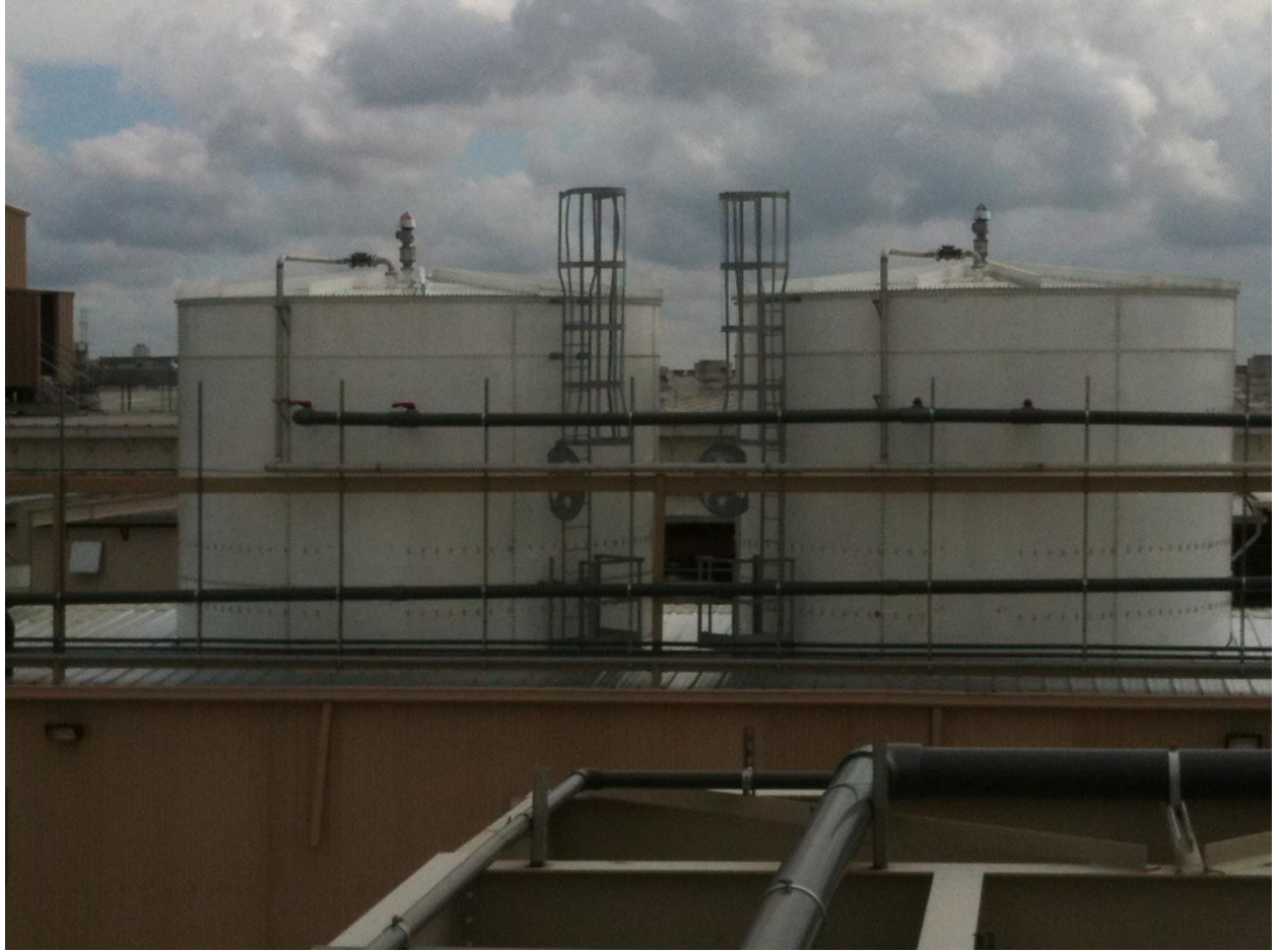
Figure 7. UASB anaerobic bioreactor tanks
